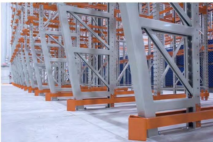
Guardrail with deflector
